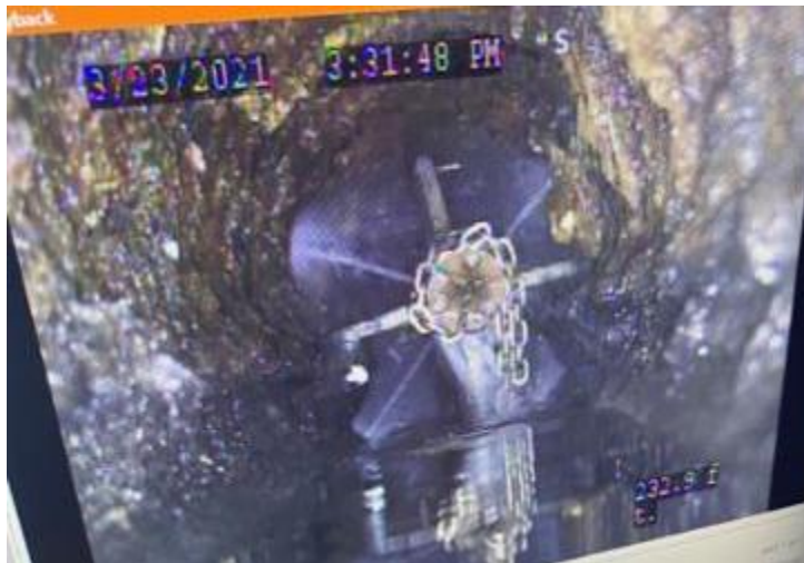
Figure 1. View of Keller Beach sewer pipe prior to cleaning. Hydro nozzle is in use. Chain flail is in view.
